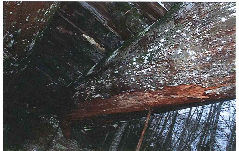
CK2232 Span 2 failed stringer
